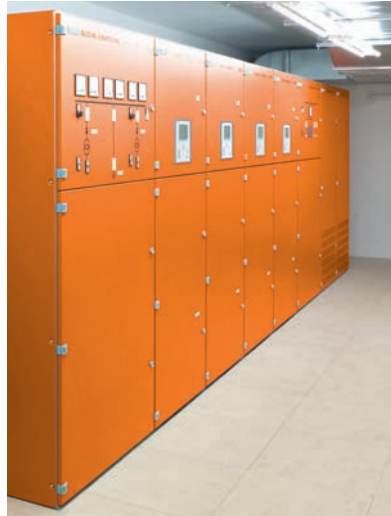
Project: Substation Hardthöhe, Fürth, Germany
