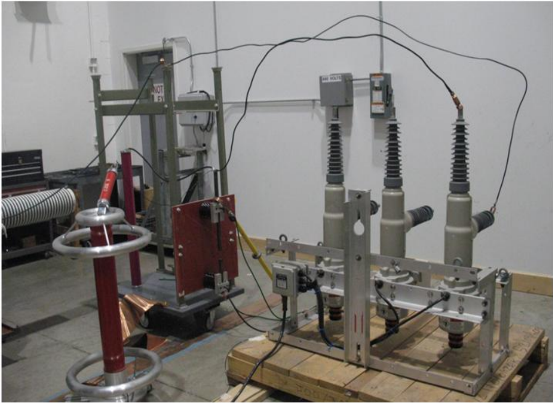
Test Setup with the recloser
