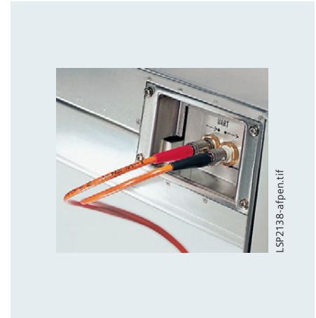
Fig. 5/36 View from below showing system interface (SCADA) with FO connection (for remote communications)
