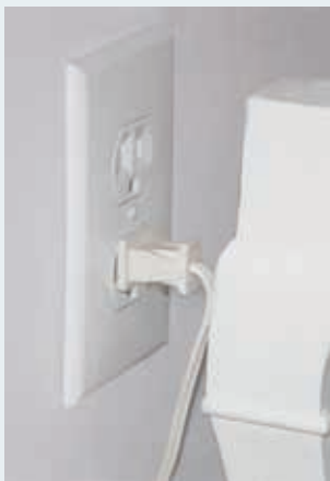
Damaged power supply cord
