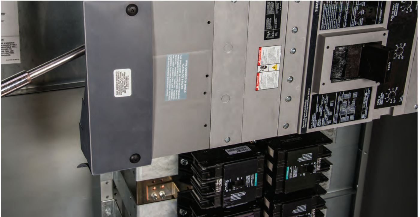
ND Main Breaker (With line side UL 67 barrier installed on the left side of the breaker)
