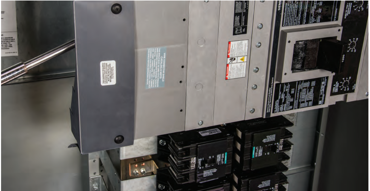
ND Main Breaker (With line side UL 67 barrier installed on the left side of the breaker)
