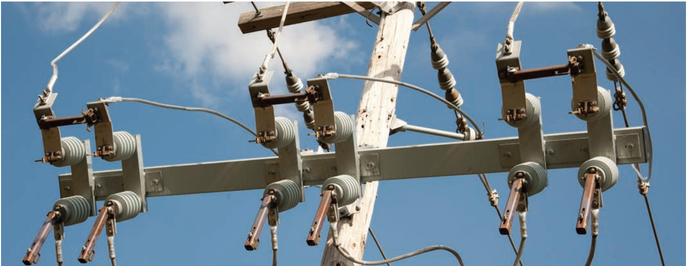
Figure 2: B-2 installation three-pull bypass
