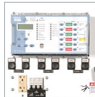
Type 7SR224 control and protection relay (triple-single)
