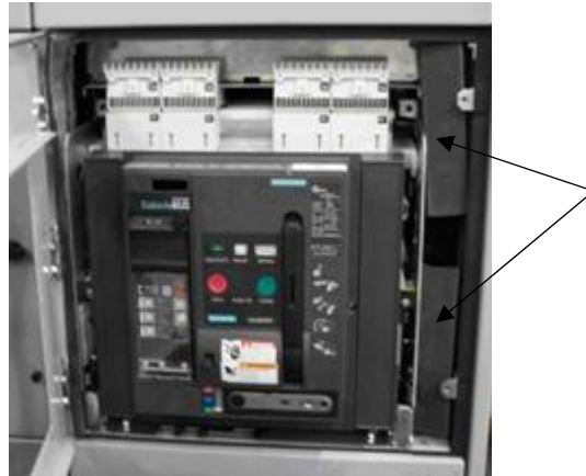
Figure 4: Front View of Breaker Compartment
