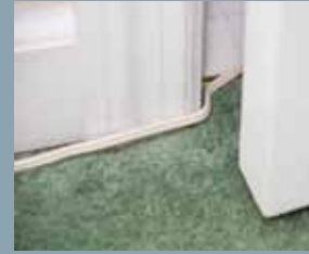
Damaged power supply cord (Example: door continually "pinches" cord)
