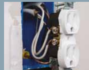
Screw terminal where a wire is connected to a receptacle may become loose as it is pushed back into the work box
