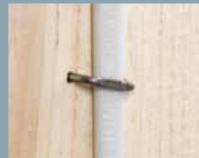
Hammering electrical cable staples too tightly into studs during rough wiring
