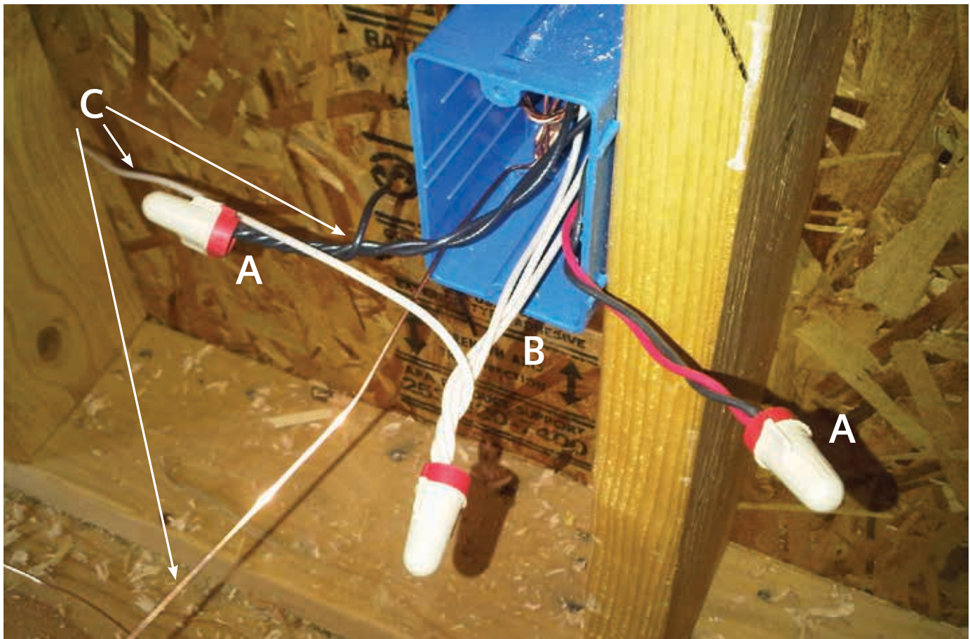
Figure 1: Multi-wire branch circuit junction box with load connections accessible
