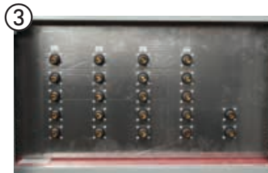
3 2000A example of Crouse-Hinds Cam-Loks for a three phase four wire system with ground connections
