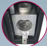
Control Wire Taps
