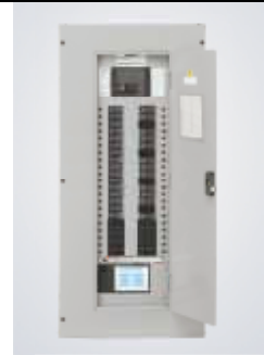
i-3 Lighting Controls
