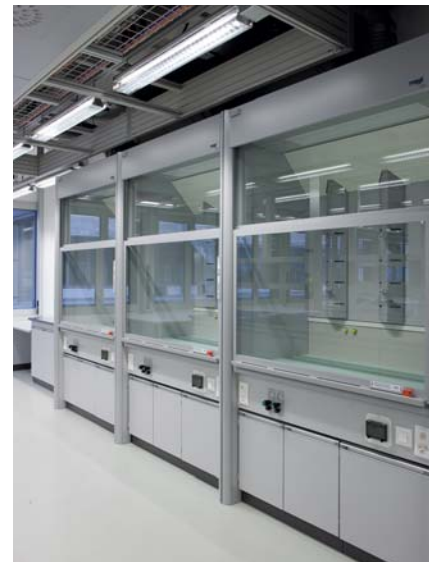
Fume hoods at Dow Europe in Horgen, Switzerland
